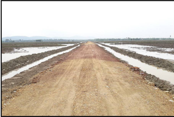
Construction of farm road in Kawt Kha Mel village of Mawlamyaing Township
