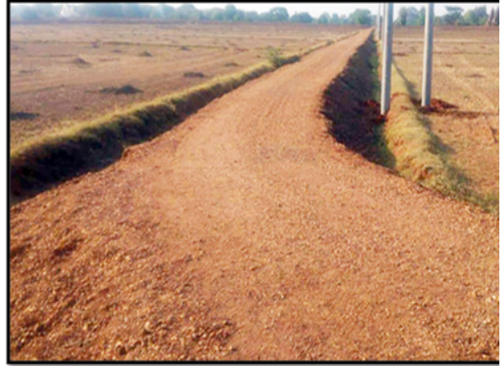
Construction of farm road in Myin Kyun-Inn Gone village of Magway Township
