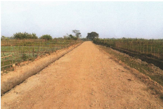
Construction of farm road and its bridge in Phayar Paung village of Kyauktaw Township
