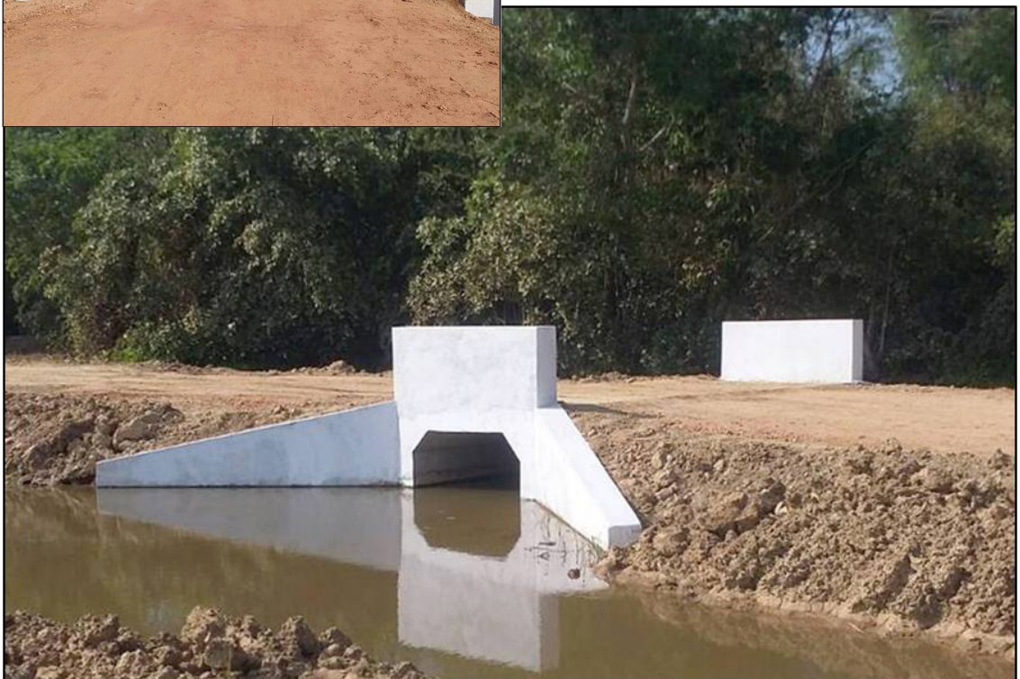
Construction of farm road and its box culvert in Tharyar Kone village of Tike Gyi Township
