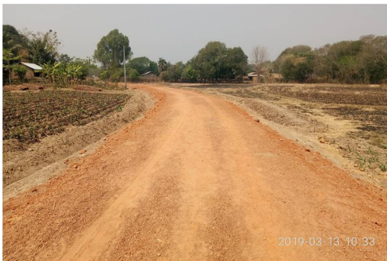
Construction of farm road in Thike Kyin Ma village of Pauk Khaung Township
