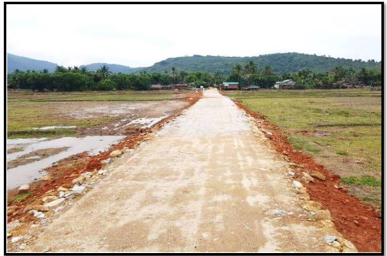
Construction of farm road in Sam Hla Kone village of Ye Township
