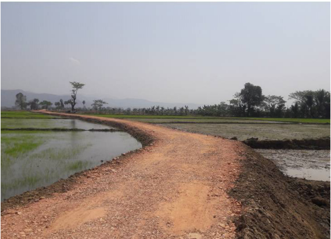
Construction of farm road in Yone Pin Village of Lewe Township (Earth+ Gravel)
