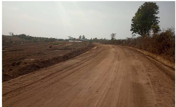
Construction of farm road in Poe Sar Tau village of Ottarathiri Township
